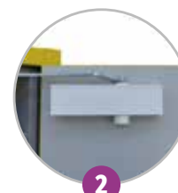
Self-closing doors with thermo-fuse
